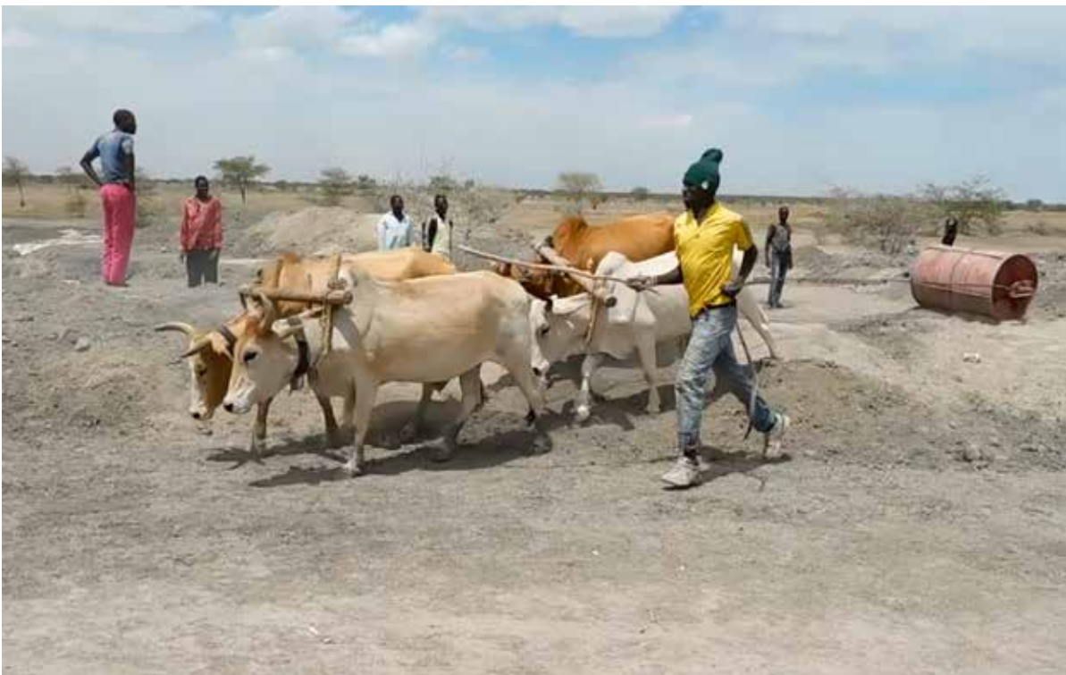
Figure 3: An ox-drawn compactor was built out of an old oil drum and is used to compact the embankments
