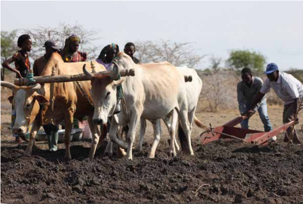
Figure 2: An ox-drawn scoop (locally constructed) is used to remove the soil from the excavation area and dispose it where the embankment will be established.
