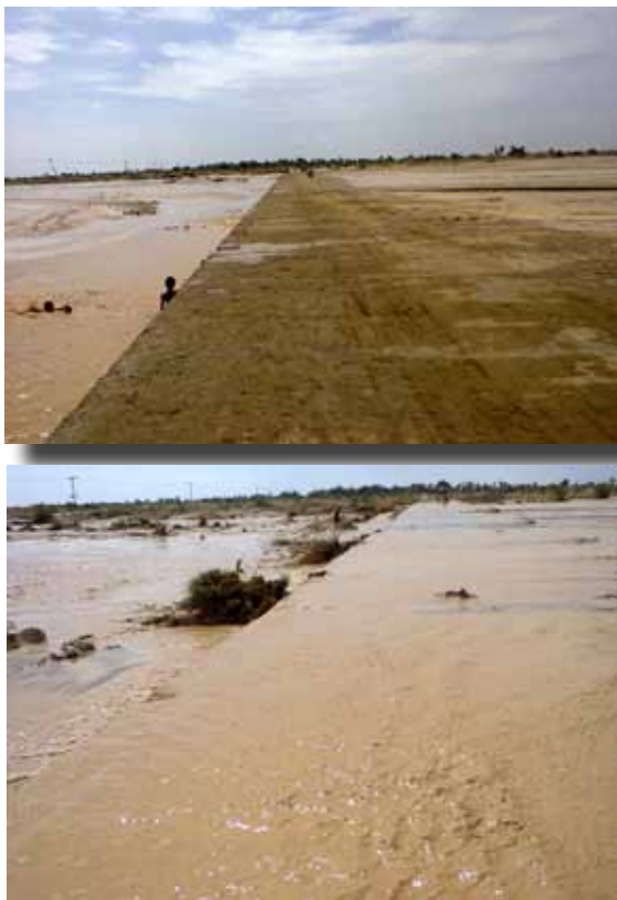
Figure 4: Road crossing at Kot Kaisrani (Pakistan), the upstream riverbed is stabilized with the construction of a drift
