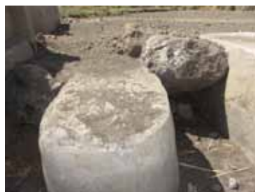
Figure 3: Large boulders blocked scour sluice gate (Libsekal et al., 2014)
