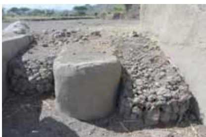
Figure 2: Farmers intentionally blocked scour sluice gate with gabions (Libsekal et al., 2014)
