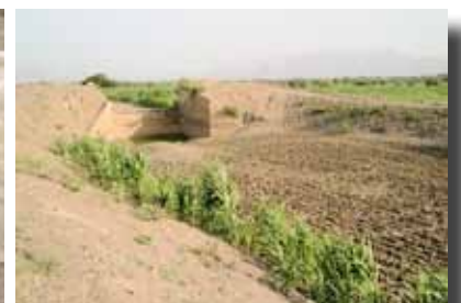
Figure 4: Huge sedimentation made drop structure redundant (Ratsey, 2011)
